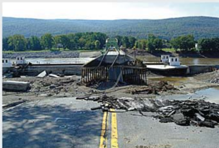
River bridge destroyed by heavy flooding.
